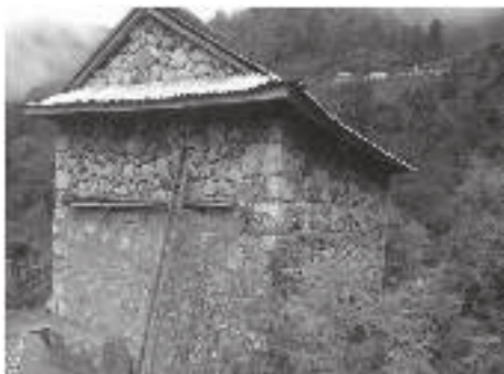
Fig. 15. Masonry building with no gable band.
