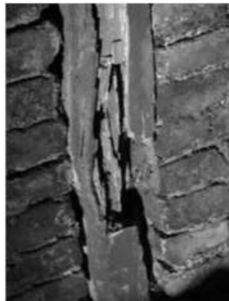
Fig. 22. Decayed posts of ground floor.
