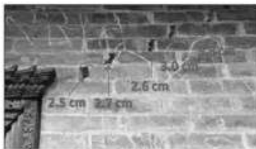
Fig. 26. Cracks in the external wall of ground floor. (Source: (Wood, et al.))
