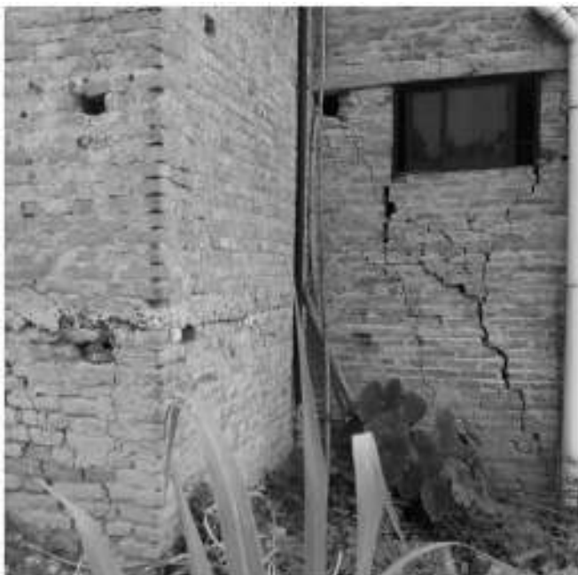
Fig. 7. Crushing of bricks of external wall.
