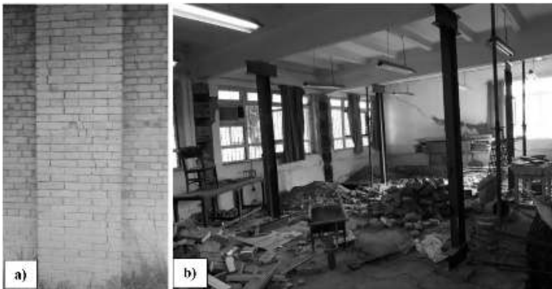
Fig. 4. a) Brick cracking in compression and shear in the pier b) View of precast beams which are directly resting over brick piers and precast slab panels resting on beams.
