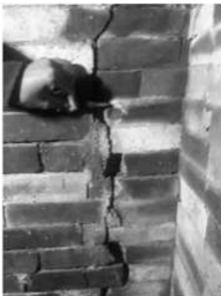
Fig. 25. Cracks in internal walls of ground floor.
