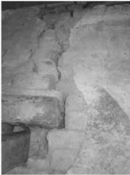
Fig. 19. Cracks in first floor.
