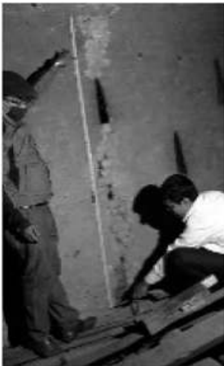
Fig. 20. Cracks in second floor.
