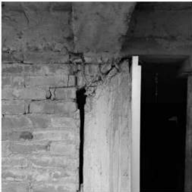
Fig. 4. Shear failure of column.
