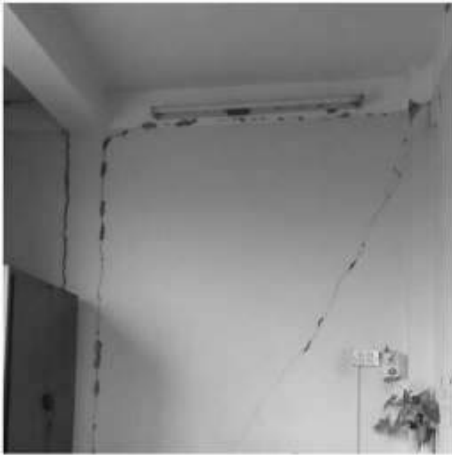
Fig. 6. Cracks in wall column interface.
