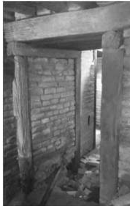
Fig. 21. Decayed posts of ground floor.
