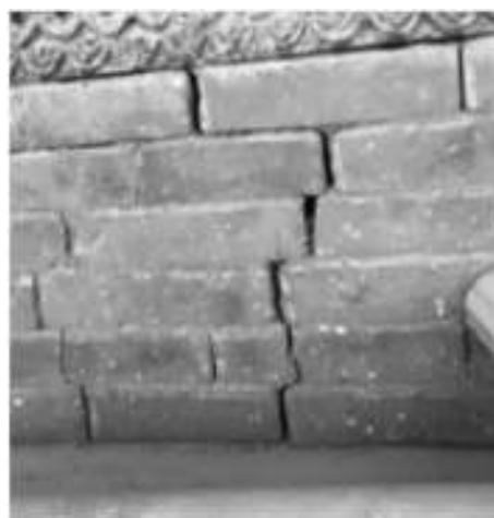
Fig. 27. Surface cracks in second floor.
