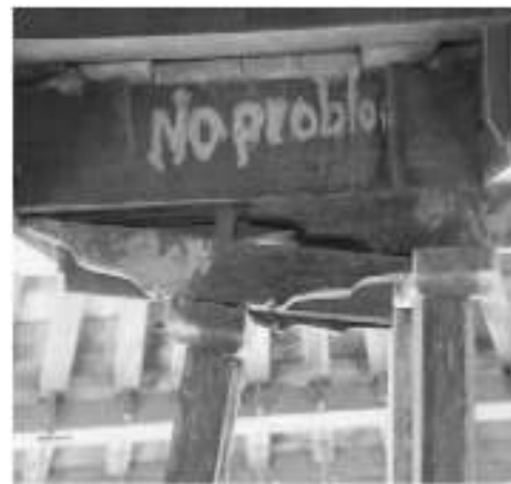
Fig. 18. Dislocation of posts.
