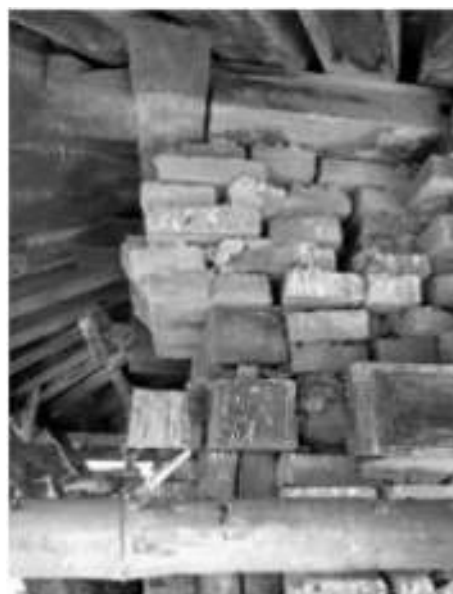
Fig. 28. Damage in the top floor.
