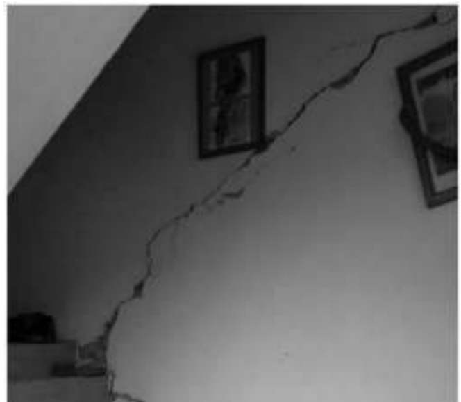
Fig. 5. Diagonal crack in staircase wall.
