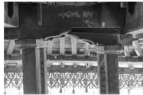
Fig. 17. Tilting of posts.
