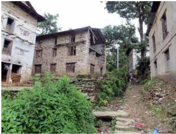
Picture 9: Vernacular buildings of Dwalkha damaged by the earthquake
