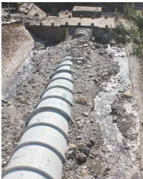
Figure 34: Damaged penstock pipe of Upper Bhote Koshi powerhouse. View to W
