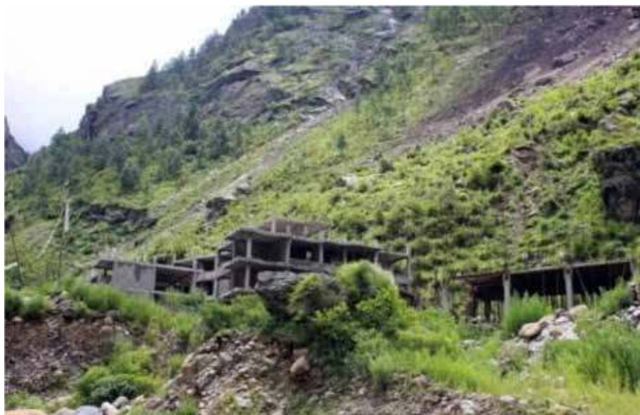
Figure 17: Buildings of Rasuwa Gadhi Hydropower Project damaged by rock fall. View to E
