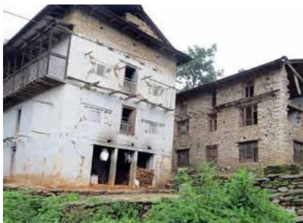
Picture 8: Houses damaged by 2015 earthquake
