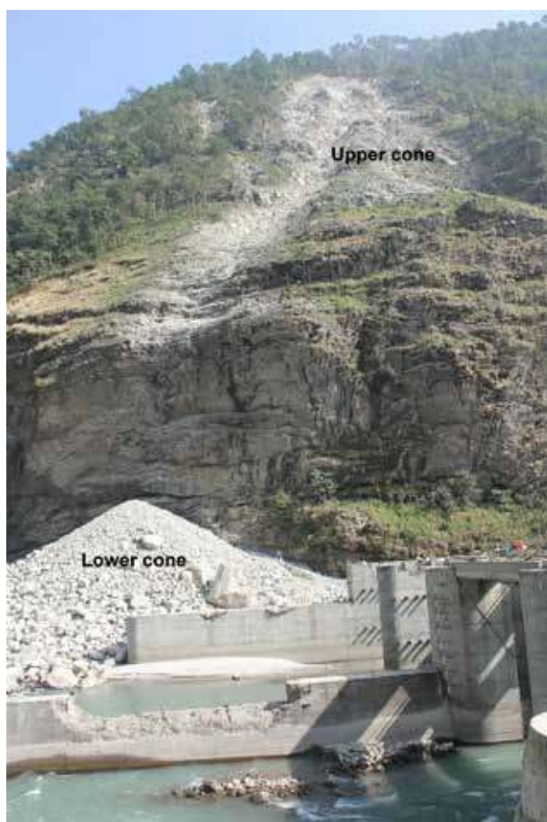
Figure 22: About 150 m high rockslide–rock fall with a large talus cone on left bank of Trishuli River. View to E
