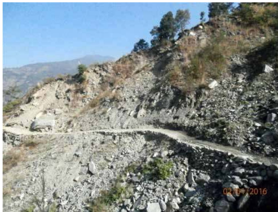
Figure 14: Dharna colluvial slide affecting Dundure–Dhading Bensi road
