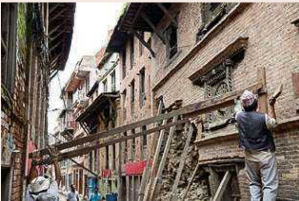
Photo 7: Supporting damaged houses. (Source: kvptnepal.org)
