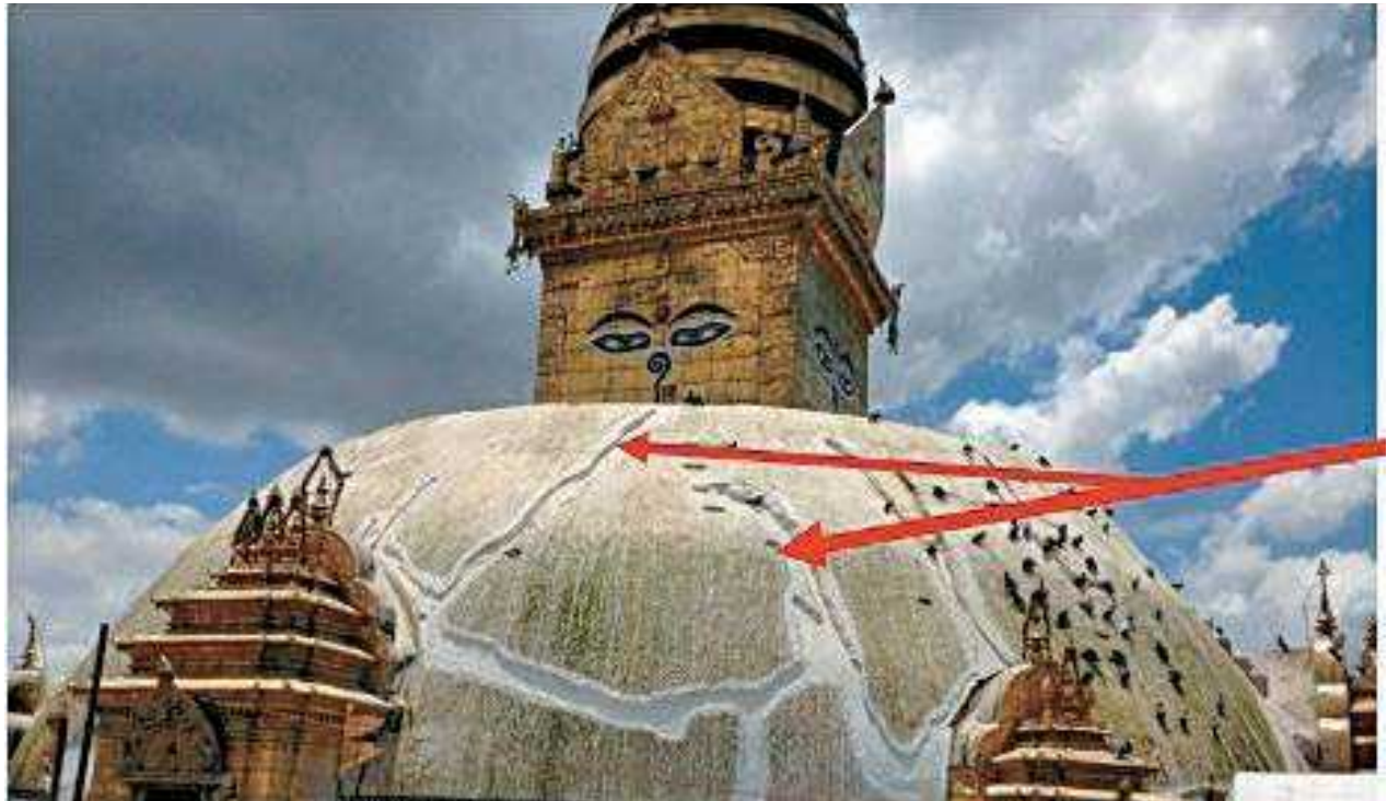
FIGURE 31: DAMAGE TO SWAYAMBHUNATH STUPA DOME STRUCTURE DUE TO EARTHQUAKE (CRACKS HIGHLIGHTED BY RED ARROWS)
