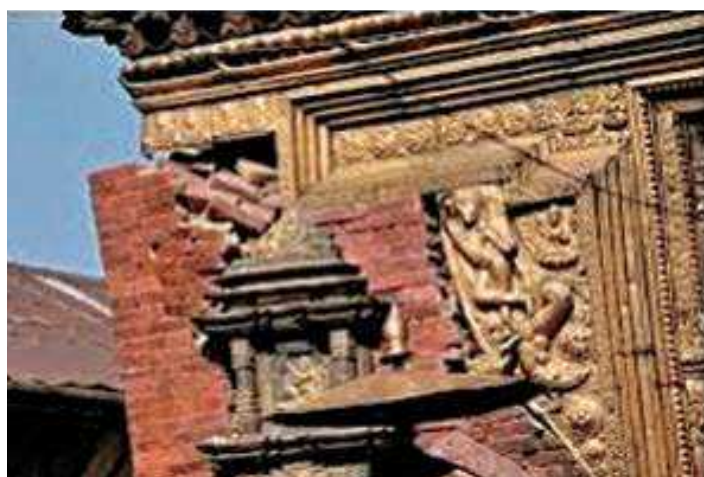
Cracks in corner wall of temple
