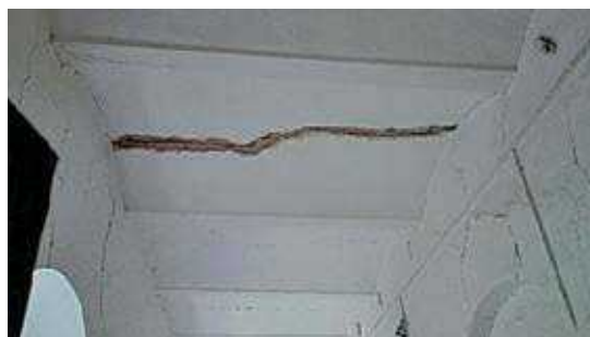
Damage in Vault Arch
