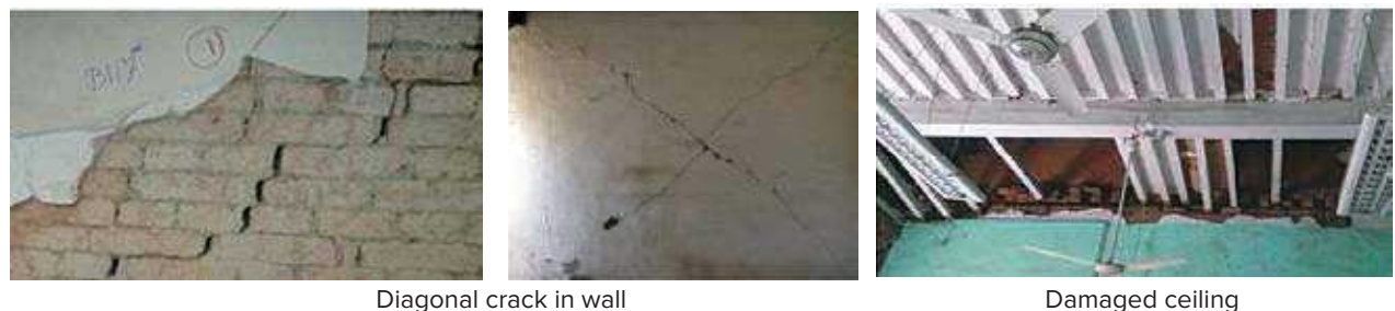
FIGURE 45: DAMAGES AT BABAR MAHAL PALACE CAUSED BY THE EARTHQUAKE
