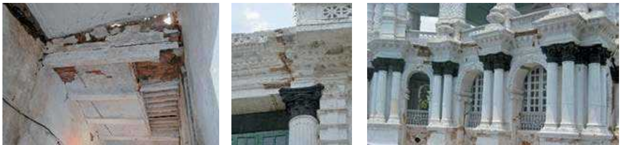
FIGURE 36: DAMAGES CAUSED BY THE EARTHQUAKE
