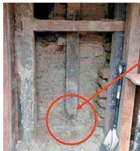
Decayed timber post inside wall
