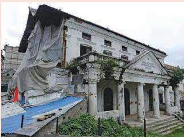
Photo 41: Durbar High School after the earthquake (Source: The Himalayan times published on Aug 20, 2016)
