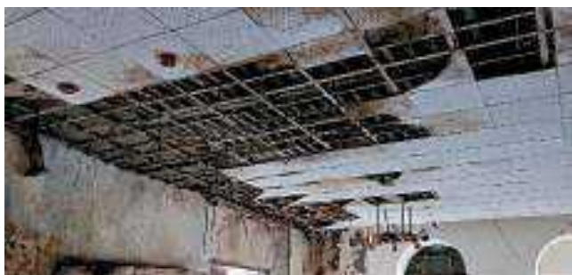
Damage in ceiling
