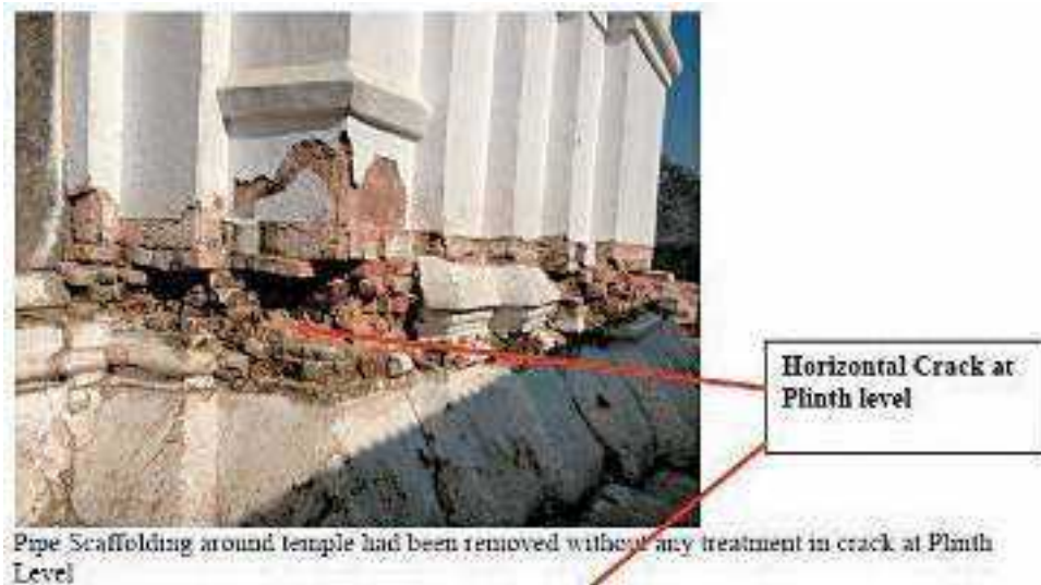
FIGURE 32: DAMAGE TO ANANTAPUR SHIKHARA TEMPLE IN THE SWAYAMBHUNATH
