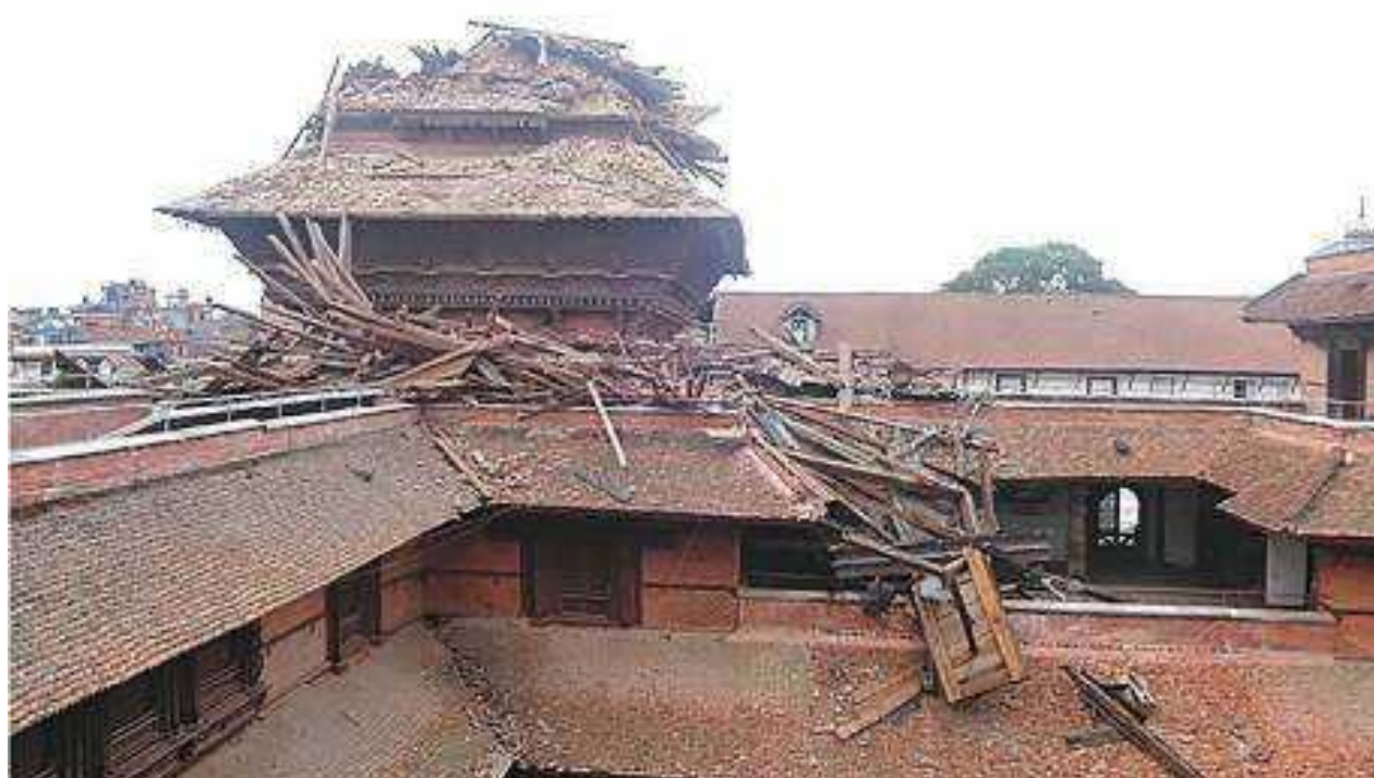
FIGURE 57: DAMAGE TO THE STRUCTURE OF THE TOWER COMPLEX
