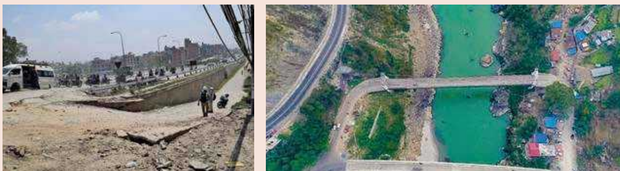
Photo 44: Example of damaged road in Kathmandu (Photo: Rama Mohan Pokhrel, 31 May 2015) and road bridge connections
