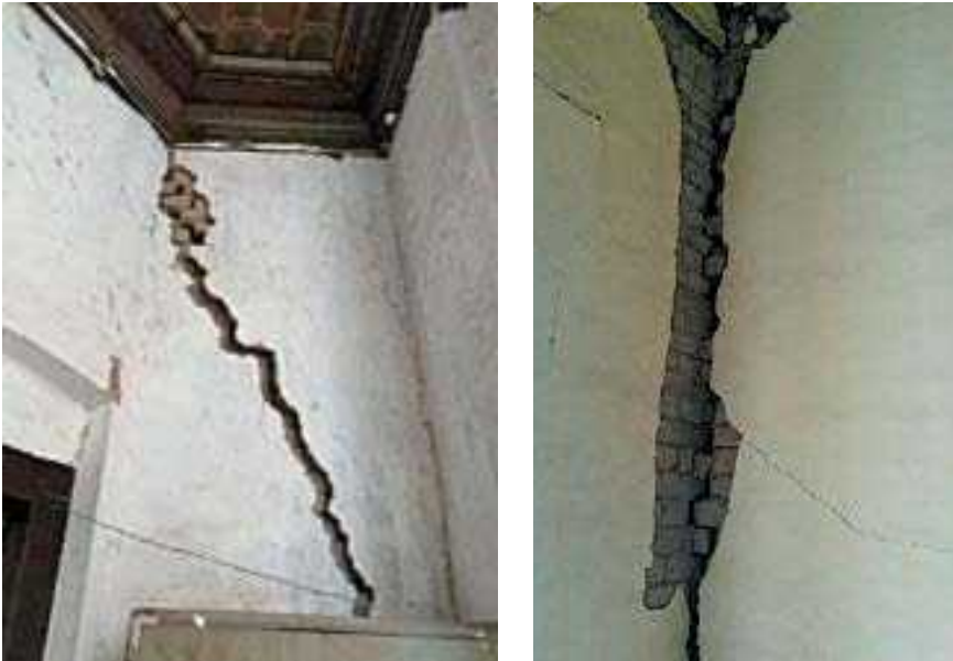
FIGURE 48: DIAGONAL AND CORNER CRACK IN THE WALL
