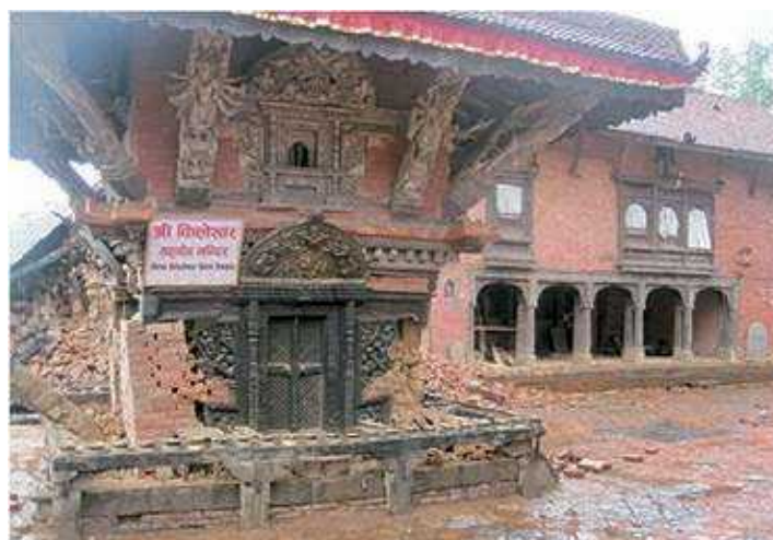
Cracks in corner wall of temple
